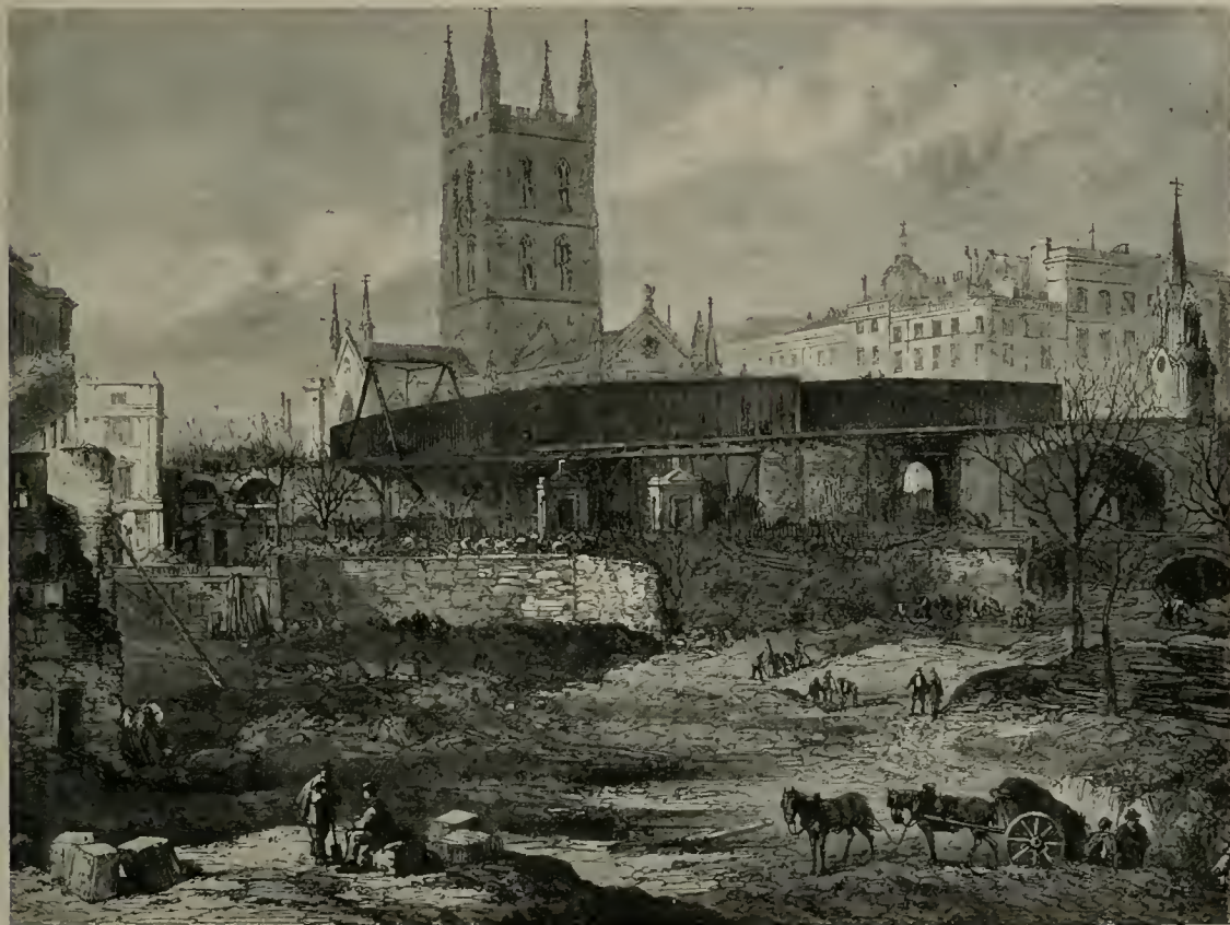
PART OF THE SITE OF ST. THOMAS'S HOSPITAL AT SOUTHWARK BEING CLEARED FOR RAILWAY PURPOSES
